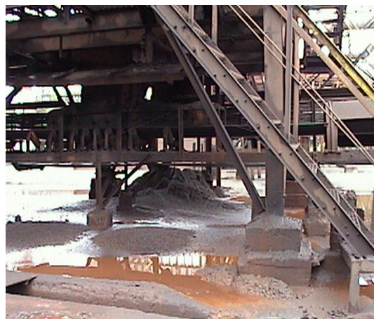
Figure 2. Spillage due to improper transfer design.
