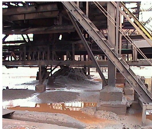
Figure 2. Spillage due to improper transfer design.
