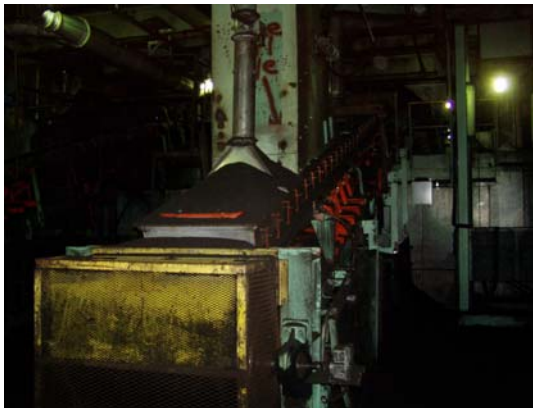
Figure 5. View of discharge portion of original transfer at Ontario Power.
