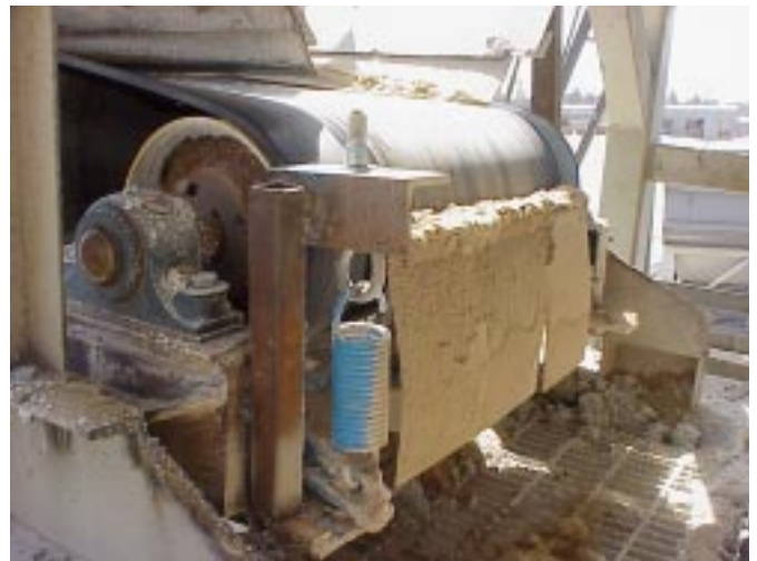
In rest position outside the kiln, slinger head-end shows why stainless steel blade-tip shields are needed to keep buildup off cleaner-blade mounting bolts for easier blade replacement.
