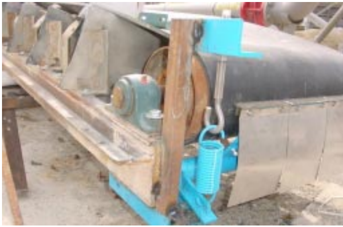
Installation of Flexco Eliminator® H-Type® high temperature belt cleaner at the head pulley of a moveable slinger shows tungsten-steel blades mounted higher than usual, with cross-pole blade mount and spring tensioning mechanism trimmed to fit within slinger's moving inner carriage.
